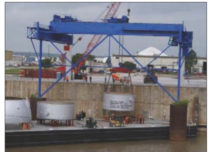
The crane has two trolleys mounted on a fixed frame
