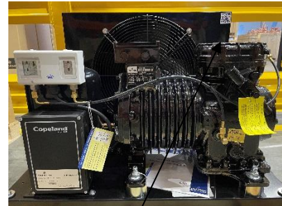
On Condensing Unit
