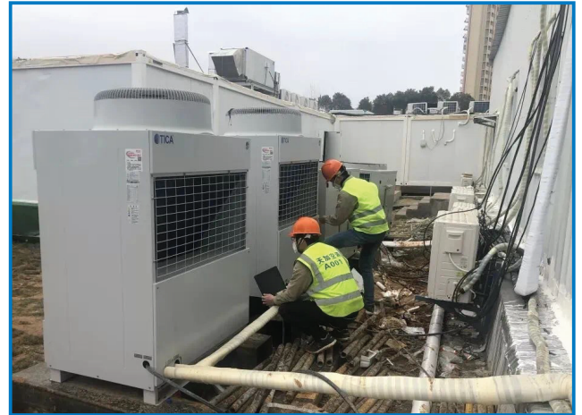
Emerson Copeland Digital Scroll™ compressors were equipped in the air conditioning systems for Huoshenshan Hospital
