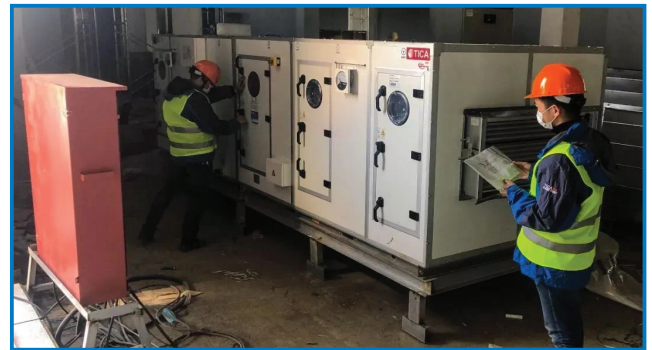
TICA setting up the medical purifying air conditioning equipment for Leishenshan Hospital
