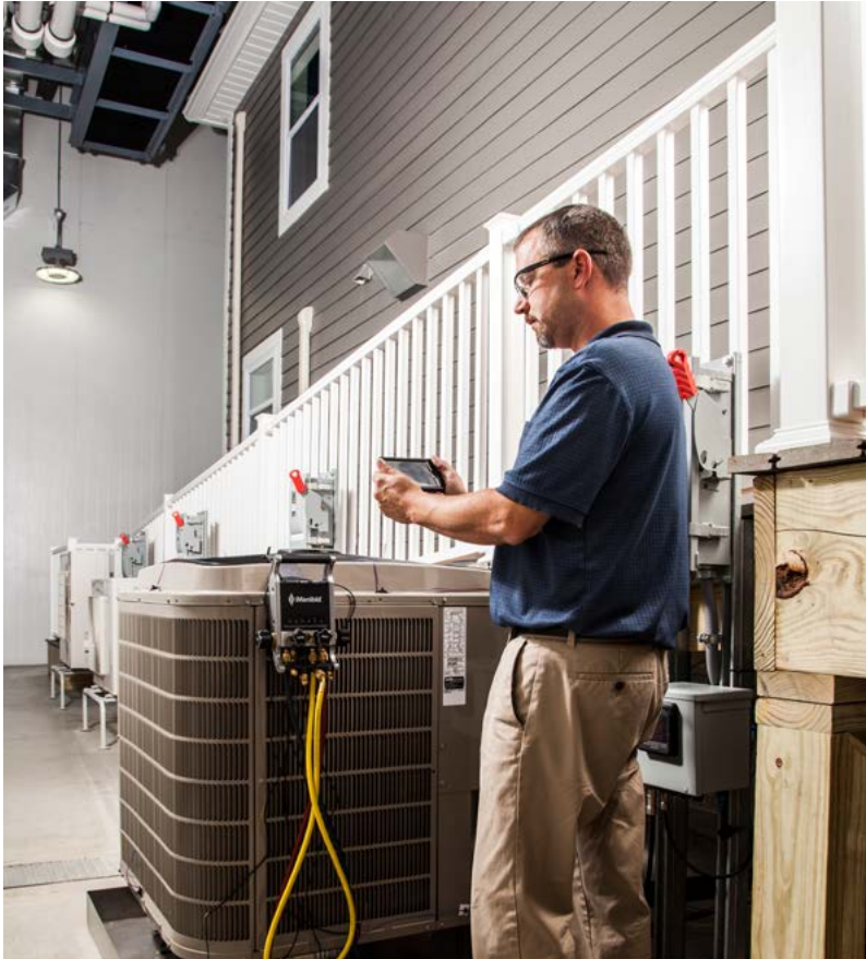
A fully functional house is built inside a climate-controlled hangar sealed with heavy doors. Large heating and cooling systems simulate the sun’s effect, allowing researchers to study the home’s energy performance on a single day in climate’s like Alaska, Arizona or Florida.
